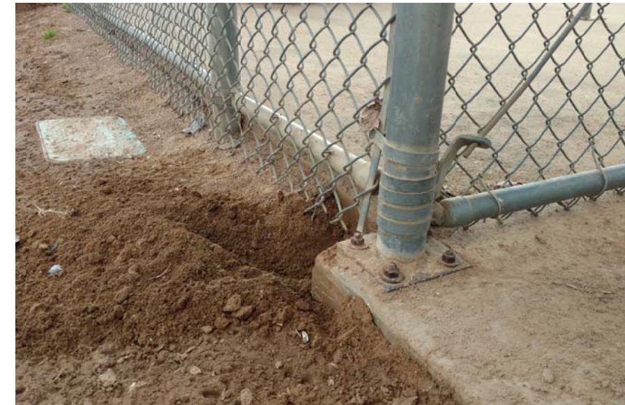
Photo of Offset in Concrete Along Field
