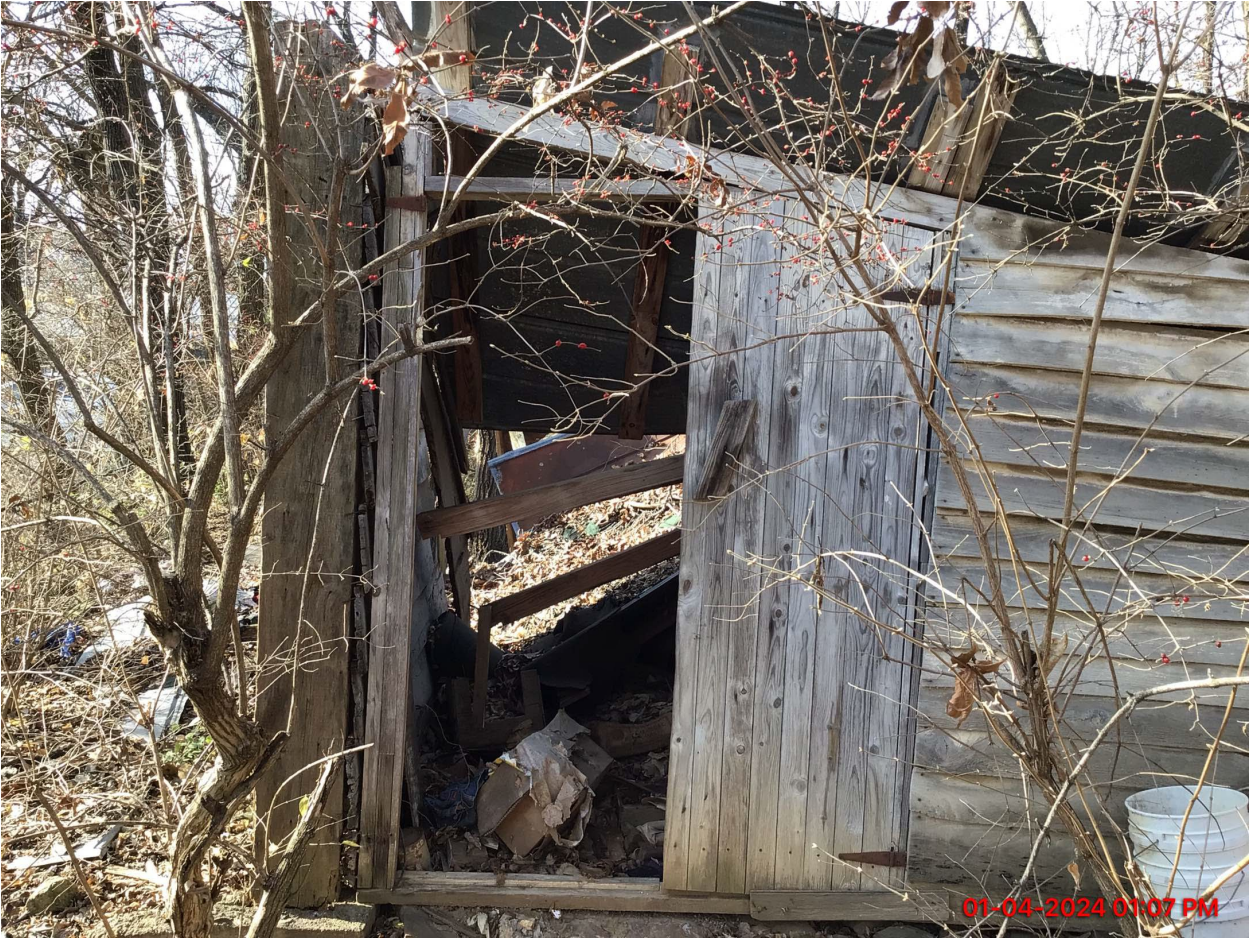
Photo of a neglected accessory building.
